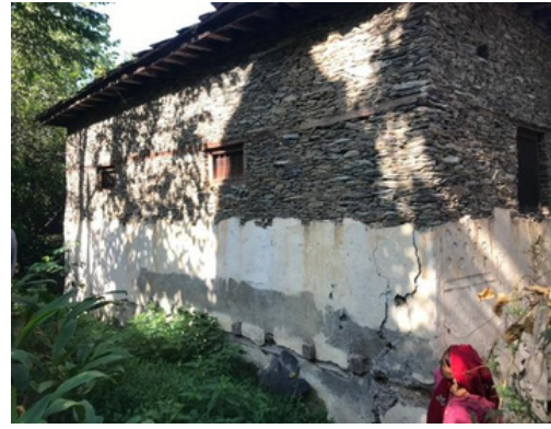
Buildings with timber bands performed well
