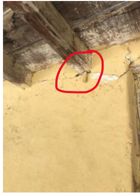
Wooden pegs in beam and wall connection to restrain the horizontal movement
